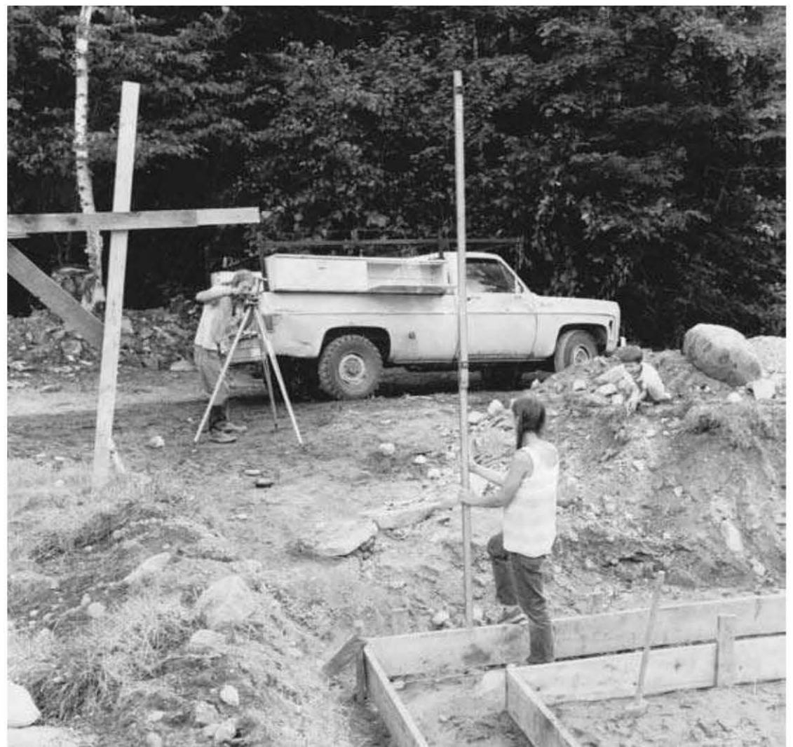
Fig. 3.11: Jaki holds a grade stake while a friend uses a contractor's level to assure that the inner and outer footing forms are all at the same grade.
