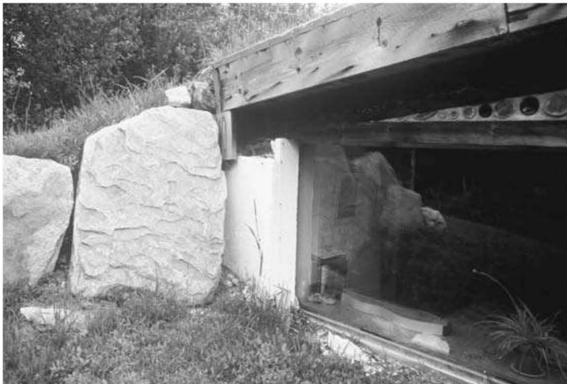
Fig. 11.1: ENERGY NOSEBLEED – TWO Rigid foam on the exterior of the exposed block wall slowed heat loss to the exterior and kept the internal wall temperature above dew point. In May of our first year in the home, we began to notice condensation around the base of the block walls. Because of the so-called “thermal flywheel” effect, the earth’s temperature in May and June is still quite cool at six feet of depth. This “coolth” is conducted through the footing to the area where the poured floor meets the block wall. Warm moist interior air hits the wall, followed by: dew point, condensation, damp. The condition was the result of our failure to insulate right around the footings and under the floor.
