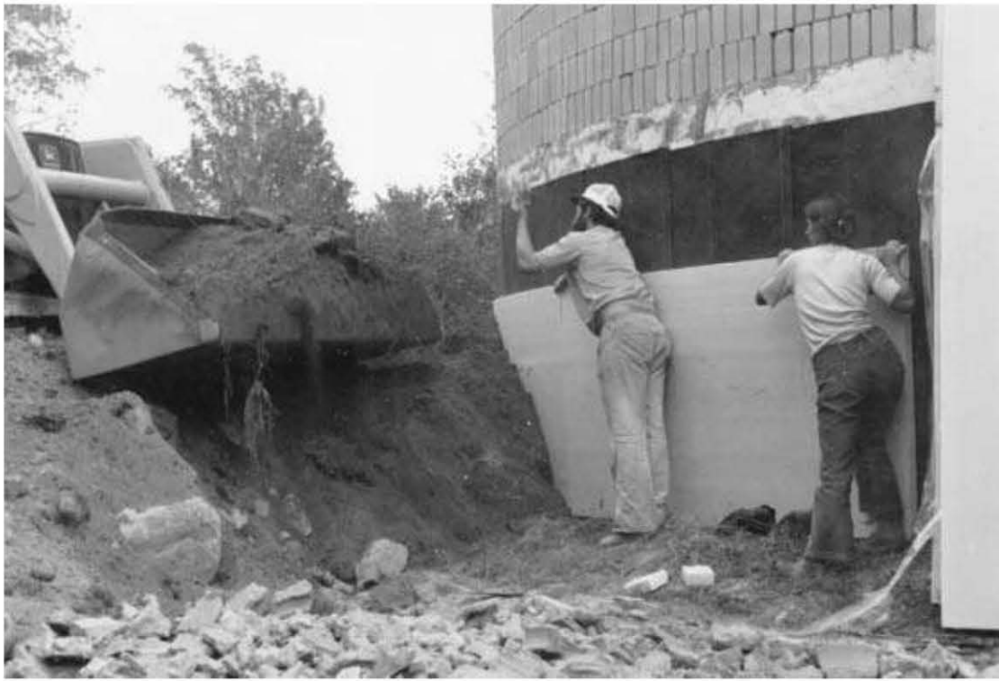
Fig. 7.10: “Bituthene ® Protection Board Adhesive” for applying lightweight protection boards, such as extruded polystyrene, to the membrane. Grace stones, Jaki and Dennis hold the extruded polystyrene against the wall during backfilling.
