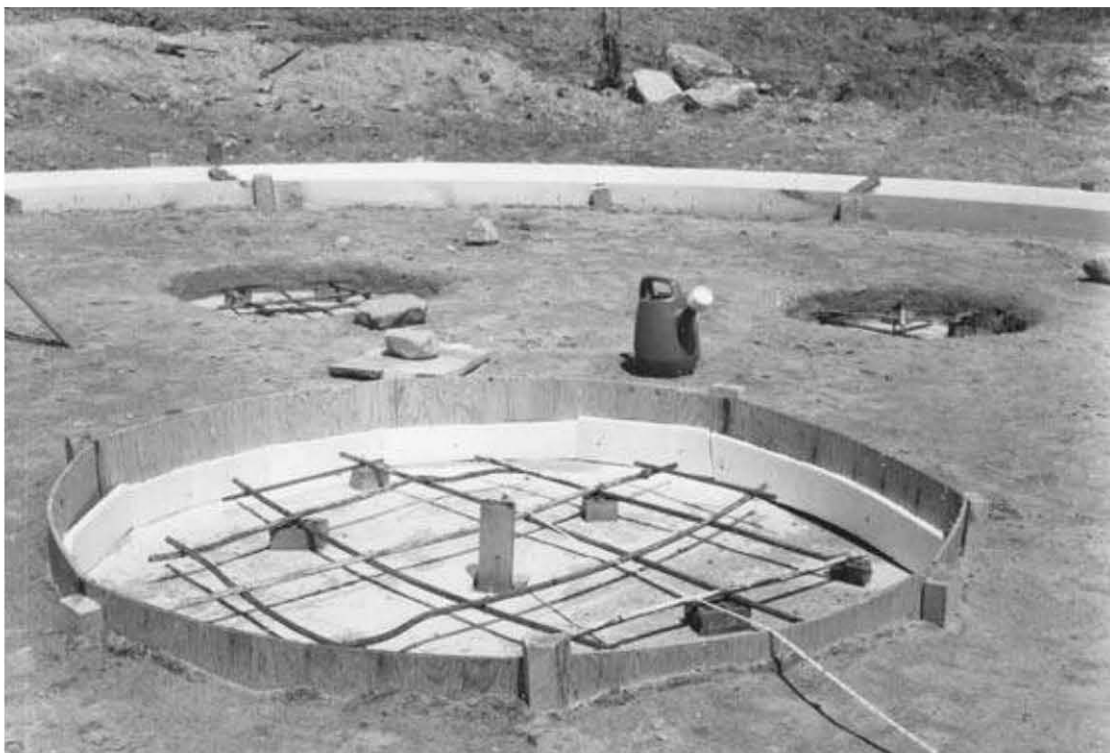
Fig. 3.21: Formed with \frac{1}{4} " plywood, the footing for the masonry stove is ready to pour.
