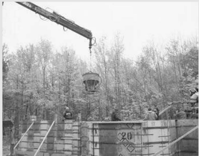
Fig. 5.1: Strong forms retain the concrete, which is delivered by chute, directly from the truck, or by hopper, controlled by the operator of the articulated boom.
