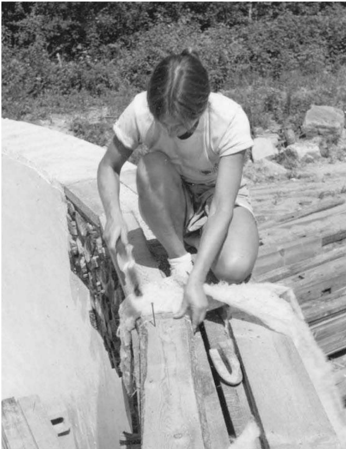
Fig. 6.16: Jaki fastens the wooden plates to the four-by-eight window lintels with 16-penny ( 3\frac{1}{4} -inch) nails. To stop draft, she has installed a strip of fiberglass insulation between the plates and the lintels.
