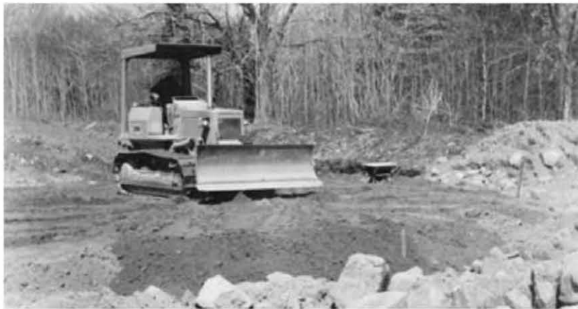
Fig. 3.5: Three or four runs of sand are built up and individually compacted, resulting in a final compacted pad of at least 18".
