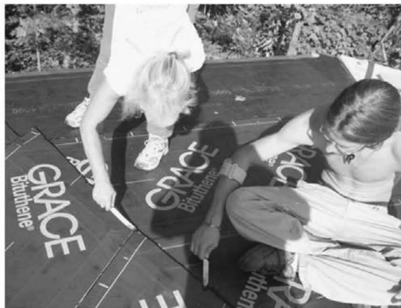
Fig. 8.3 (above): Jaki and Darin Roy feather the edge of the mastic with pointing knives, to approximate the factory edge of the Bituthene® membrane. The mastic stops the cut edge from raising up or "fish-mouthing."
